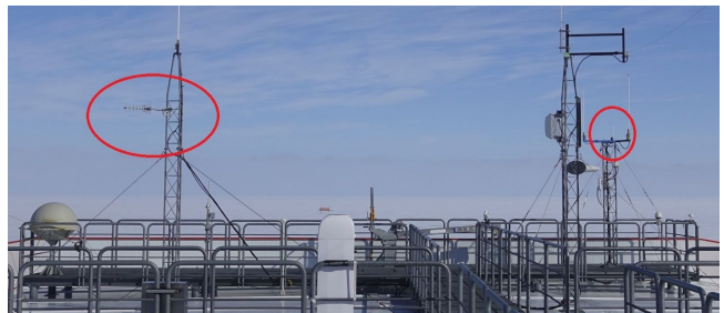
Figure 4: LoRa antennas on the roof of Neumayer III station.
